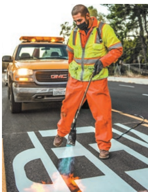
“#OurDOTCrew installed new upgrades to Balboa Blvd. in Granada Hills to keep #MovingLAFoward. High visibility messaging promotes safety for those traveling through the area.” Feb. 9
