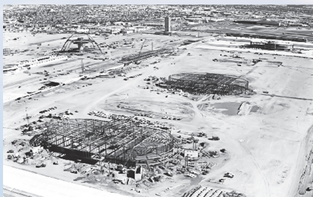
Construction was well under way for the Jet Age LAX west of Sepulveda. The Theme Building and Terminals 4, 5, 6 and 7 are visible under construction. Airports photo via the AirportHistory.org Collection.
