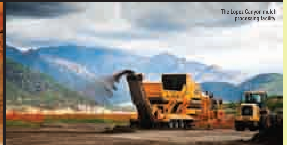
A chute collects the solid contaminants – bottles, paper, etc. – from the yard trimmings before the grinding begins.
