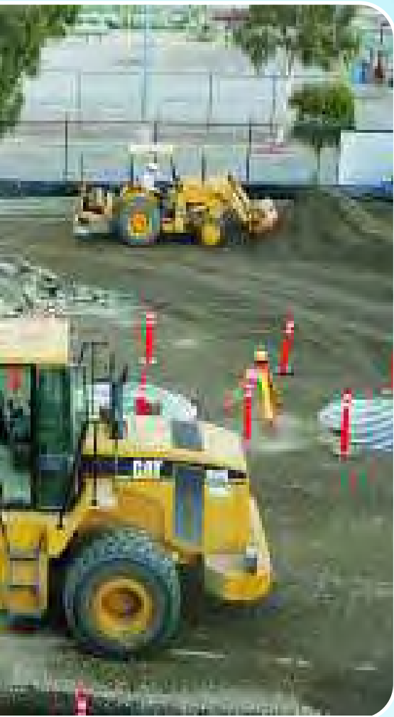
Workers have started digging the two mile-deep holes that are critical to the T.I.R.E. Project.
