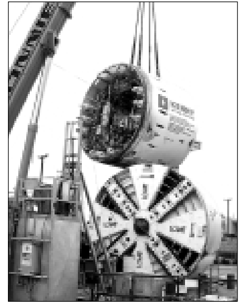
One of the four tunnel boring machines (TBMs) being used to dig the ECIS route arrives at the Los Angeles train depot from Canada, where it was manufactured. By using such technologically advanced machinery, ECIS is being built almost entirely through underground tunneling, minimizing traffic and noise impacts on neighboring communities.
