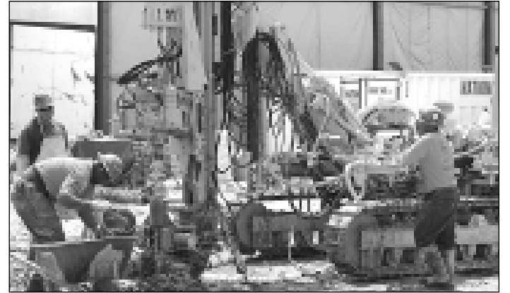
Site activity - The ECIS Construction team prepares one of the project's shaft sites for excavation.
