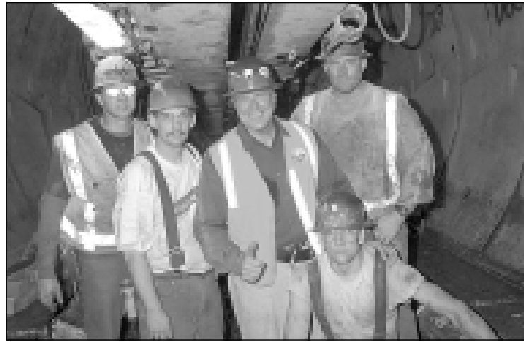
Huell Howser, host of KCET's "Visiting," with an ECIS tunneling crew. Howser recently went underground to see the ECIS construction project firsthand, and devoted a full hour to the project on his show.
