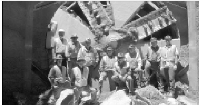
The ECIS tunnel-boring machine (TBM) named "Diane" first peeked through the shaft at Arlington Avenue and Exposition Boulevard at 11:30 a.m. May 9. No hole-through is finished without the team picture!
