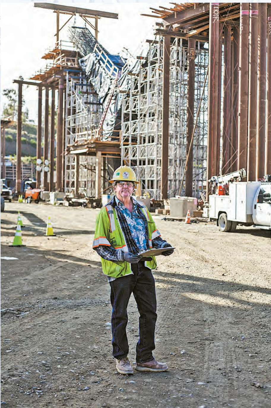
Inspecting the work is John Fitz, Construction Inspector, Public Works/Contract Administration, 4 years of City service.
