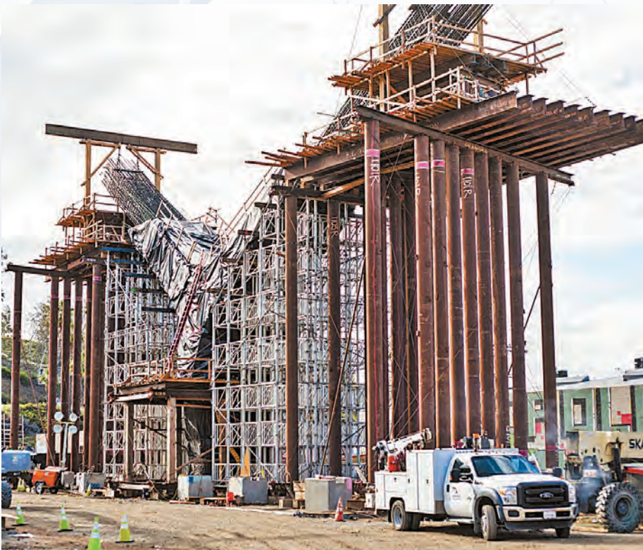
At Bent 11, workers are casting the bridge’s center column in place. At this point, the 10-foot diameter concrete foundation pile was drilled and installed approximately 160 feet into the ground, and they are raising the roadbed so it can soar over the 101 Freeway. The columns are cast in place.
