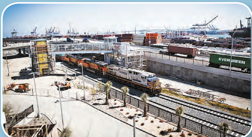
Grade separation: This new transportation overpass plays several critical roles: it flies truck and car traffic over the very busy rail line, saving sometimes 40 minutes of waits for vehicles waiting for a train to pass. This saves time and greatly reduces the burning of fossil fuel.
