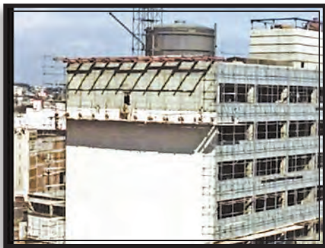
The Police Administrative Building under construction, as seen in the film shown to tour-goers.
