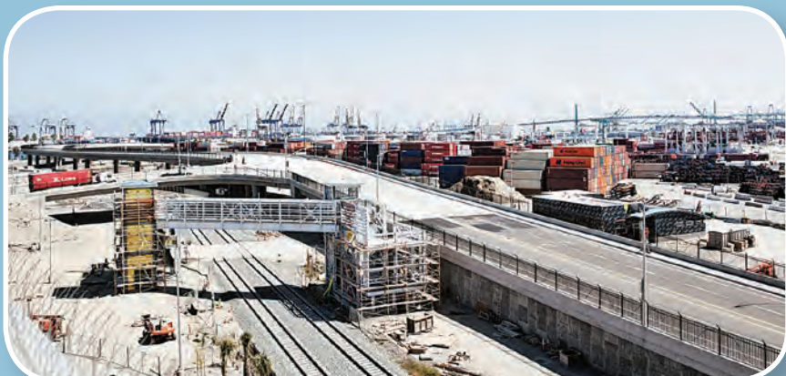
Pedestrian bridge: This pedestrian bridge will allow private-employment longshoremen to park safely in a lot waiting to be surfaced (left) and then walk from their cars and using the pedestrian bridge to walk over a passing train on their way to check in at the vendor's yard operations facility (right, not shown). The employees can cross the tracks on the ground through a safe walkway when there is no train passing through.
