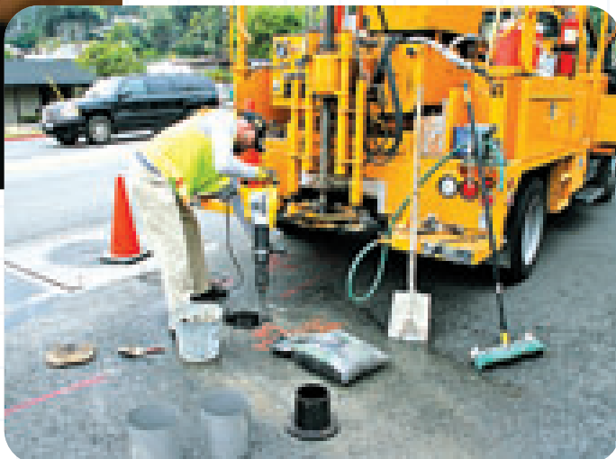
ABOVE: A Survey Division drill rig crew installs a monument into a City street.
