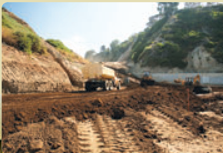
ABOVE: Many hundreds of thousands of cubic yards of dirt will need to be moved on the Potrero Canyon Project.
