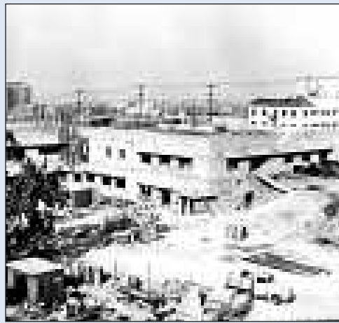
The current Central Receiving Hospital under construction in 1956. The hospital is scheduled to be razed.
