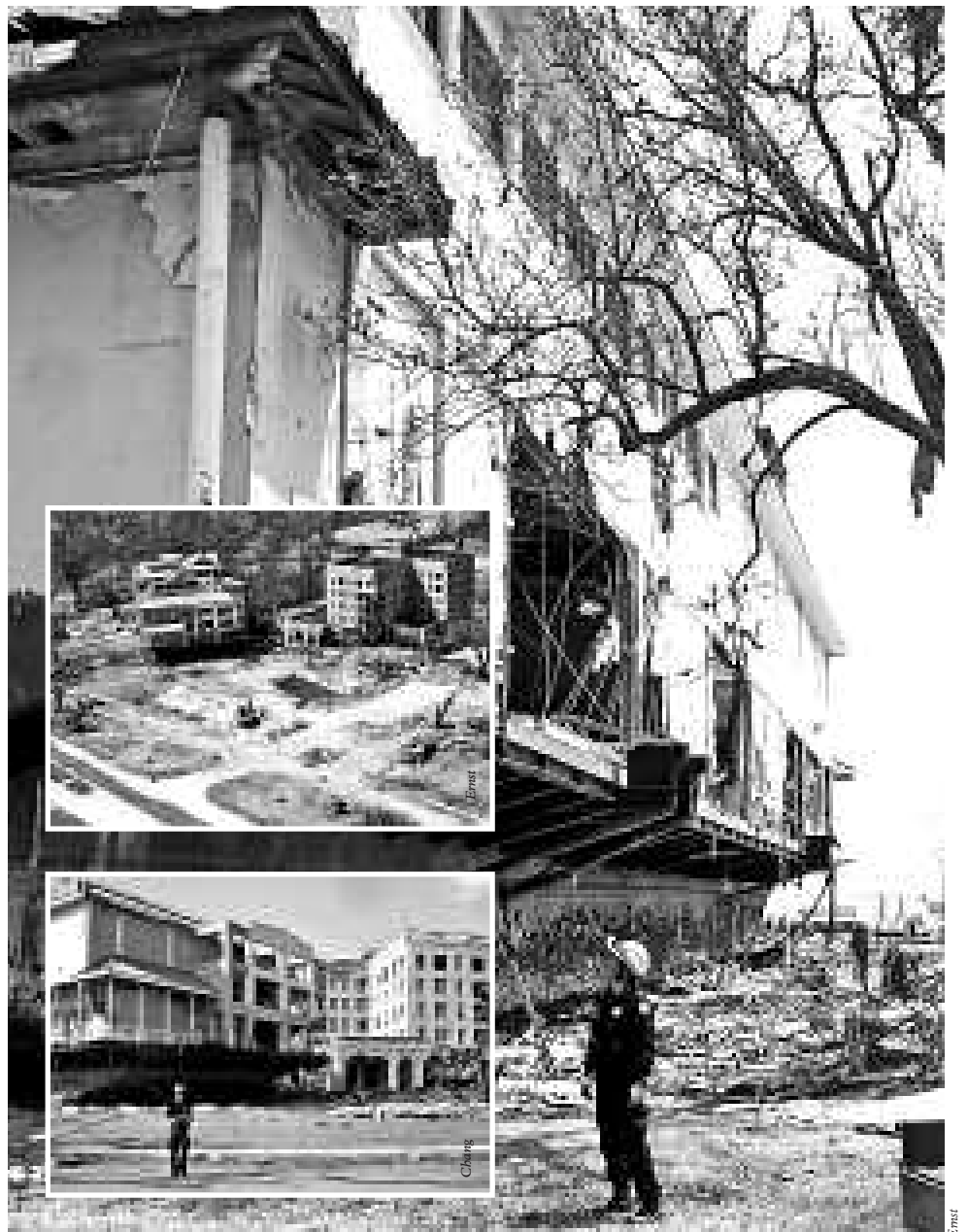
Building and Safety Structural Specialist and USAR Team Member Charles Chang stands in front of a casino barge that destroyed a two-story apartment and a five-story building (inset). LAFD Planning Manager and USAR Team Member Chris Kawai looks up to a casino barge that damaged at least two major buildings including the Biloxi Yacht Club.
