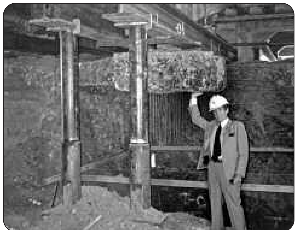
Dr. Ed Krupp pretends to be Atlas in "holding up" the old support beams during the excavation of the new Observatory space, under the building's front lawn. New support beams were put in to accommodate the expansion.
