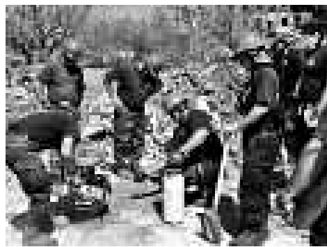
USAR Team members use a rotary saw to gain access to a lower floor. A water sprayer is used to control the dust.
