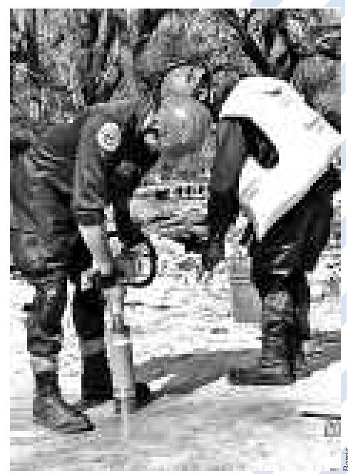
LAFD Tech Search Specialists and USAR Team Members Patrick Leising and Jerimia Spring at work in Mississippi. Patrick uses a Pomeroy to cut an access hole for the search cam. Jerimia uses a water pack to control the concrete dust.
