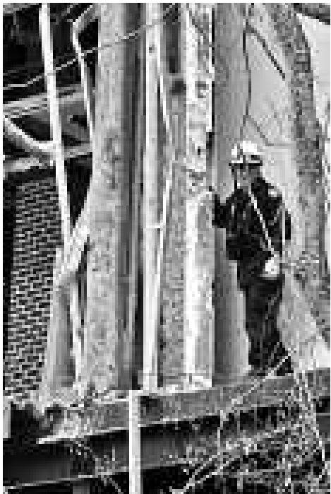
LAFD Planning Manager and USAR Team Member Chris Kawai assesses damage.
