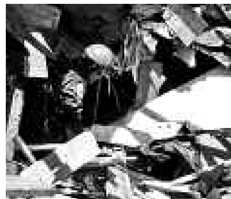
LAFD Capt. and USAR Team Member Jaime Lesenski, front, enters a collapsed structure in Biloxi, Miss.
