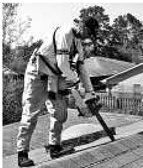
LAFD Capt. Rob Cordobes, Swift Water Team member, cuts into an attic during a search operation.
