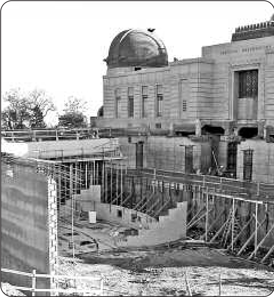
The front lawn of the Griffith Observatory was dug up temporarily to construct a major expansion underground. The lawn has since been restored. The beginning of the Leonard Nimoy Event Horizon Theater can be seen.
