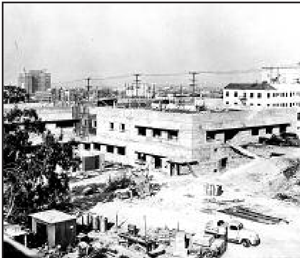
The current Central Receiving Hospital under construction in 1956. The hospital is scheduled to be razed.
