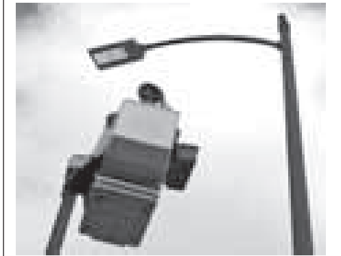
Public Works/Street Lighting's Tim Spradley inspects an LED light being tested.
