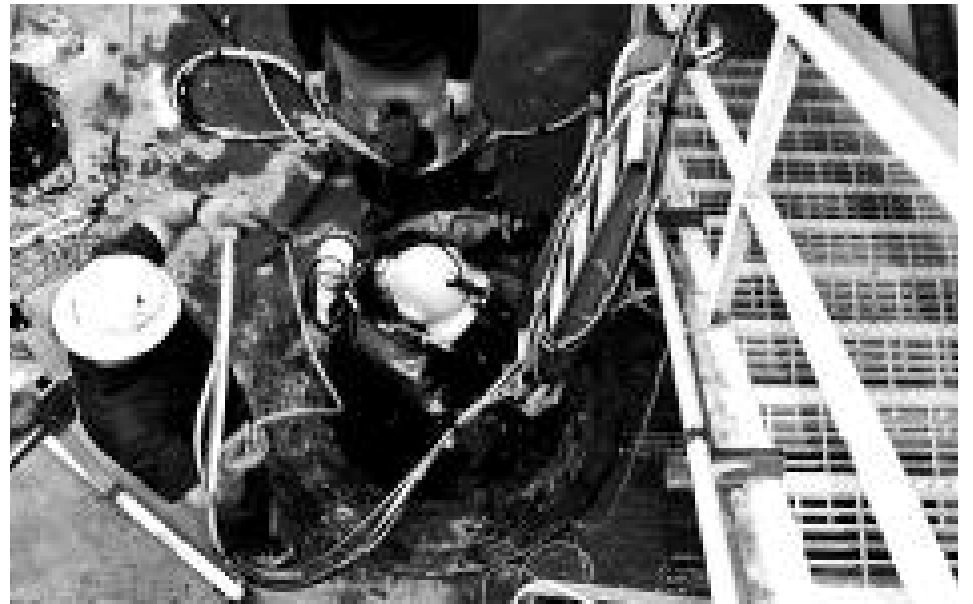
Public Works has equipment and technicians in place to gather data on the inside of the outfall.
